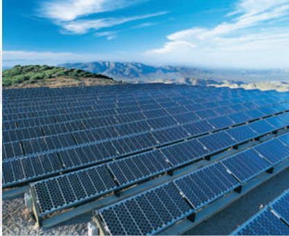
Demand for photovoltaic panels is expected to increase
