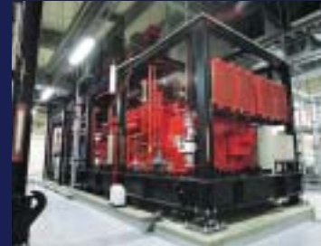
The Kyotanabe Plant's cogeneration system
