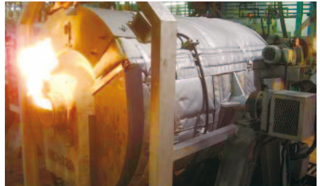
Insulating cover attached to a large-scale retort furnace
