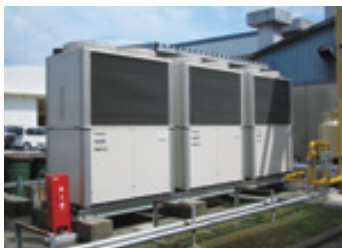
Gas heat pump air conditioning units
